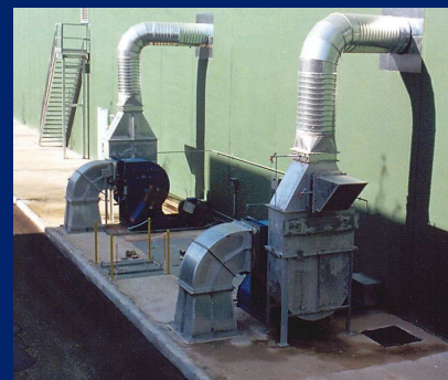
Ventilatori alimentazione biocella Biocell feeding air fan
